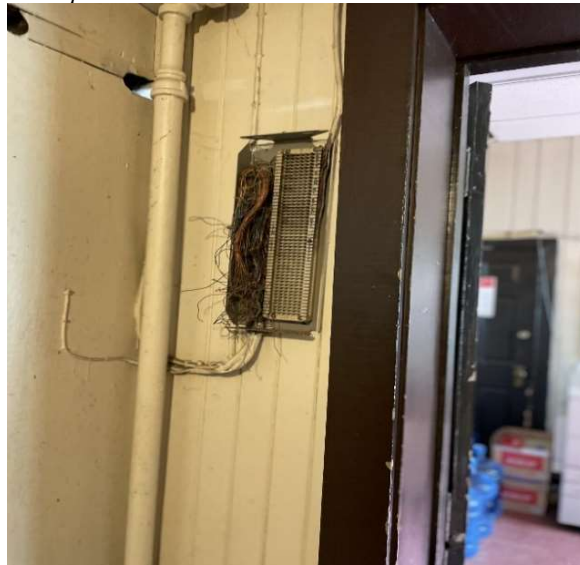
Figures 15: Wall panel with exposed wires
