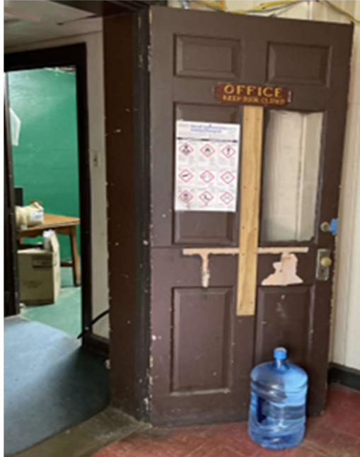
Figure 11: Broken employee breakroom door panel
