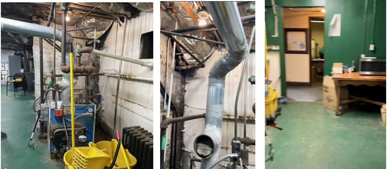
Figures 16-18: Exposed ceiling insulation in break room area
