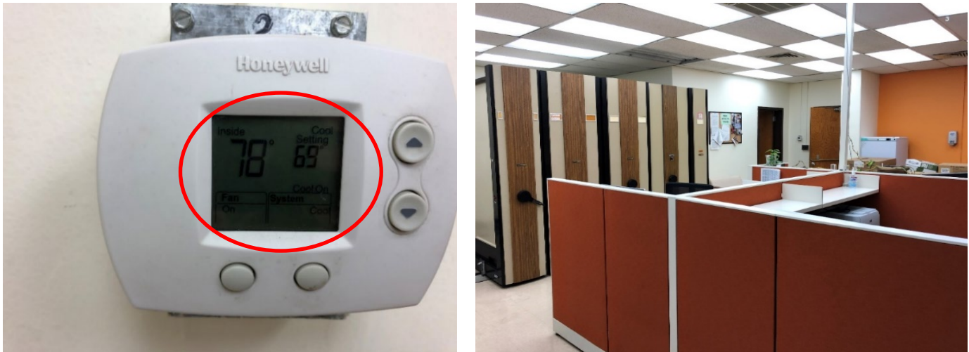
Figure 7: Room temperature higher than thermostat setting (left) and SHC staff office area where thermostat is located (right)
