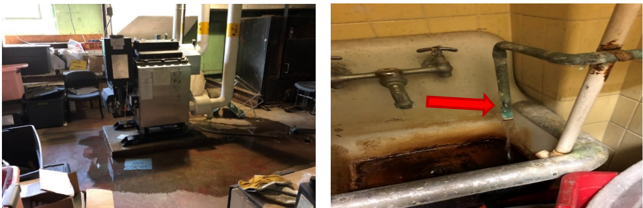
Figure 5: Water Leak in Basement (left) and running water pipe in the men's restroom closet (right).
